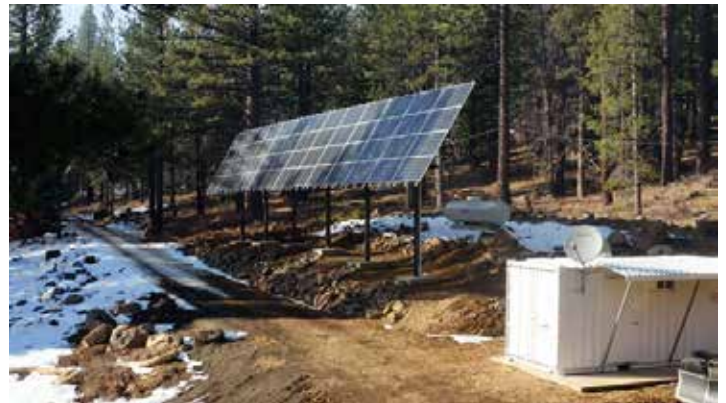
Picture of Sagehen Microgrid in California
