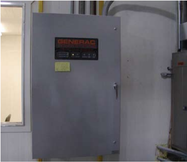
The CTTS allows seamless load transfer between utility and generator.
