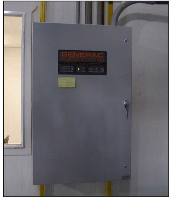
The CTTS allows seamless load transfer between utility and generator.
