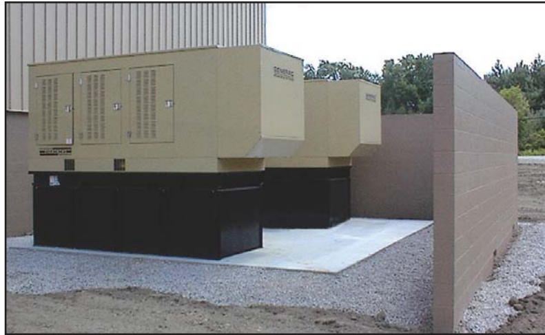
Android's two 400 kW MPS units are always standing by at its distribution center.
