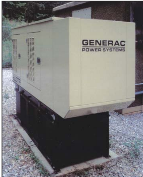
Nextel's system is more reliable because of its investment in Generac standby gensets.
