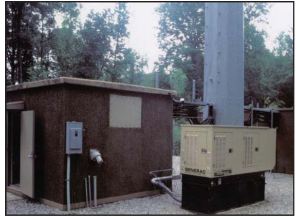
Generac is the top provider of backup power systems for telecom applications.
