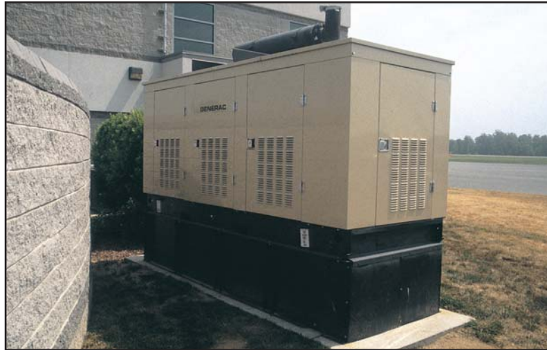
This 250 kW genset provides backup power to the airport terminal.
