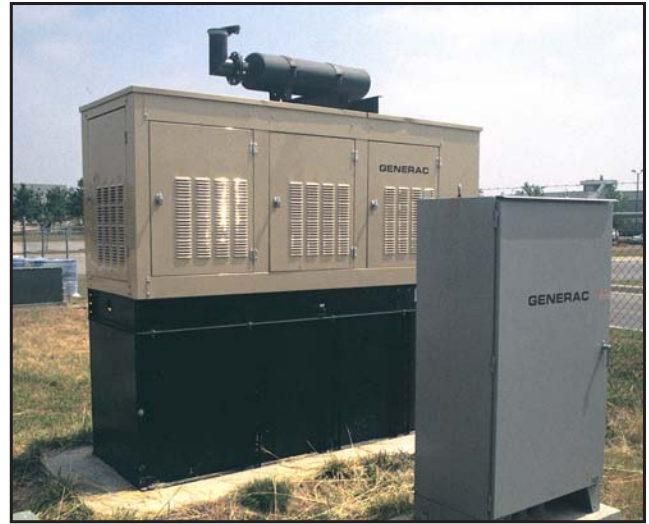
The runway lights, instrument landing system and navigational equipment are backup up by this 100 kW unit.
