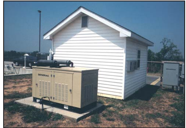
A 45 kW generator provides standby power for the fueling facility.
