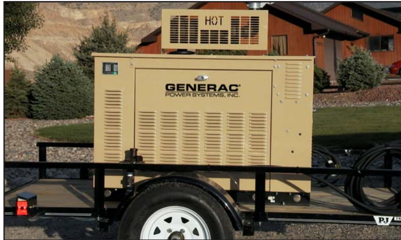
Power on the move! A 20 kW LP-fueled genset can be easily transported on this custom trailer.
