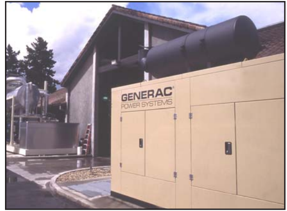
BV’s satisfaction with its smaller Generac generators led to the purchase of the two much larger generators
