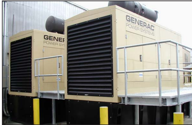
NIBCO's two 600 kW gensets keep the facility operational in the event of an outage.
