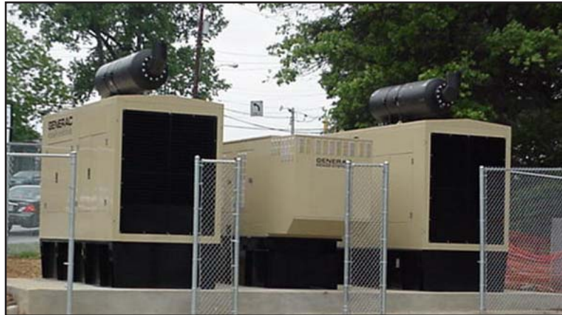
MPS flexibility is exemplified by this combination of a 400, 500 and 600 kW modular generators.
