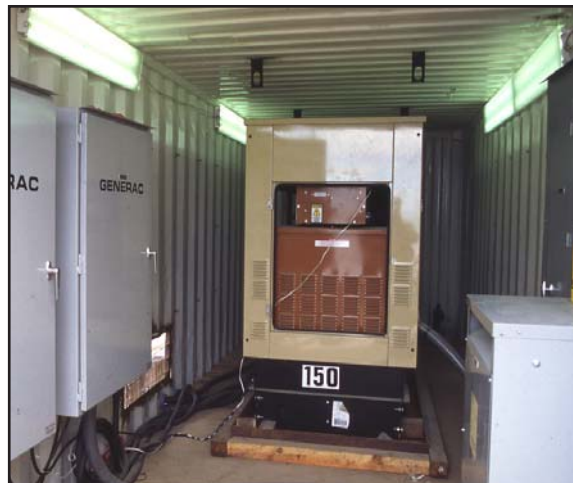
A containerized 150 kW genset.
