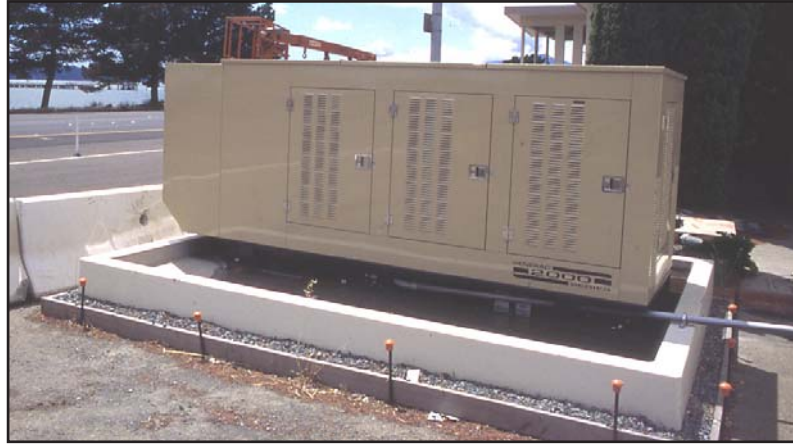
The 300 kW genset on the eastern shore is located at the toll plaza.
