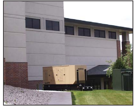
The sound attenuated genset is located alongside the building.
