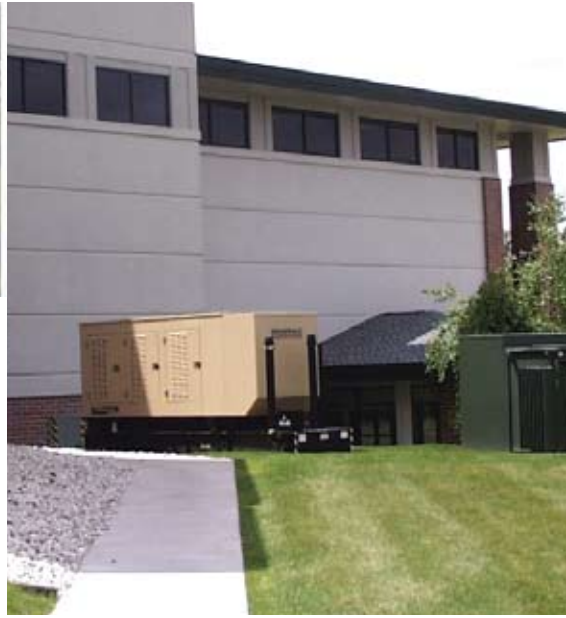
The sound attenuated genset is located alongside the building.
