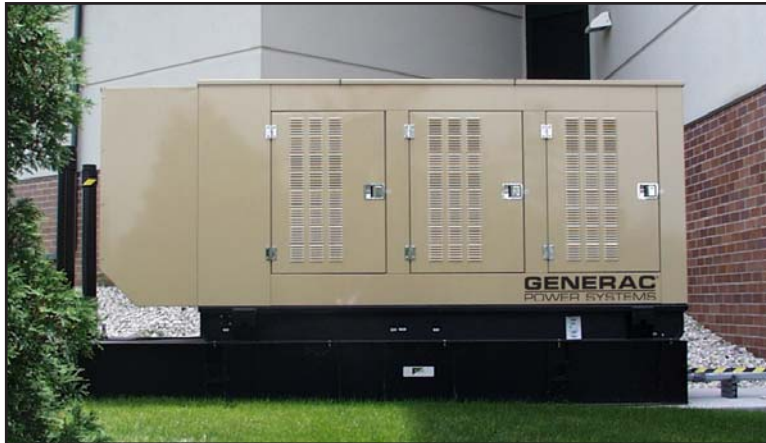
West Wood Health & Fitness Center's 180 kW genset.
