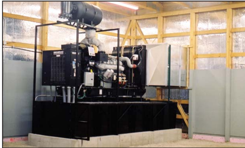
The first 600 kW MPS genset is on the job—more will be added easily, when needed.
