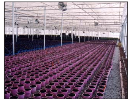
Backup power protects millions of dollars of plant inventory from the detrimental effects of a power outage.
