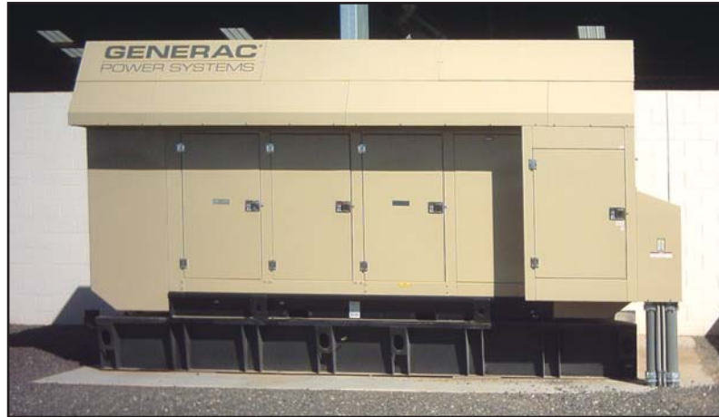
The Gemini 750 kW twin genset backs up the entire milking operation.
