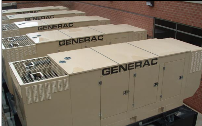
Five 400 kW gensets provide backup power with built-in redundancy.
