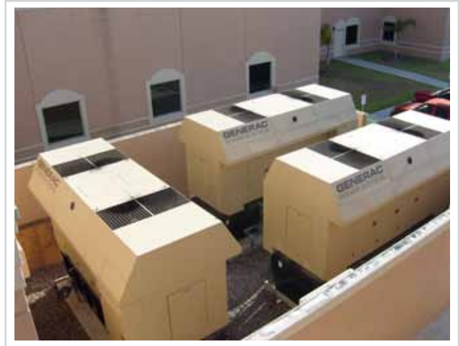
At Doctors Hospital, Generac's modular platform kept all critical systems operating for 13 straight days.
